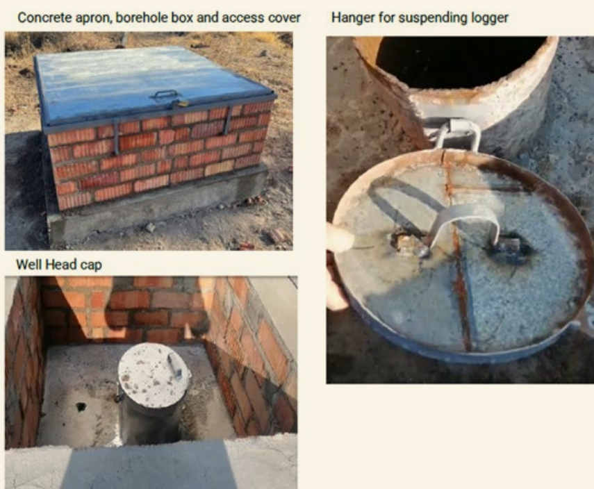
Figure 53: Example of an observation borehole with no pumping equipment. (GWR)
